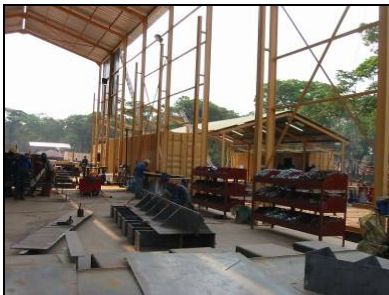
Steel fabrication work being undertaken for construction of HMS plant on site at Kinsevere mine site. (photo Oct 20, 2006)
