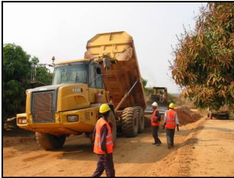
Refurbishing 27 km long access road from sealed highway to Kinsevere mine site. (photo Sept 15, 2006)
