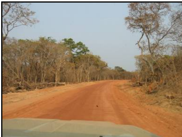
Completed section of 27km access road to Kinsevere mine site. (photo Sept 15, 2006)
