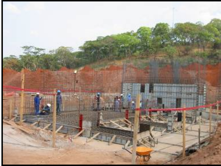
ROM Wall and crusher foundations under construction at Kinsevere mine site. (photo Oct 20, 2006)
