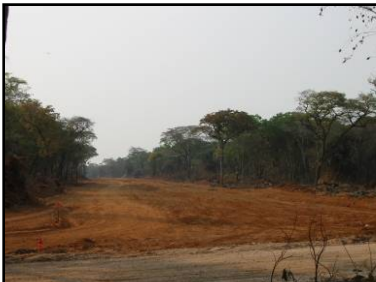
Start of access clearing for 25 kilometre long 120KV powerline to connect to DRC national hydro-electric grid. (photo Sept 15, 2006)
