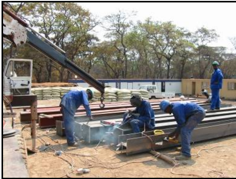
Fabrication of HMS Plant on-site at Kinsevere mine site. Construction site offices in background.
