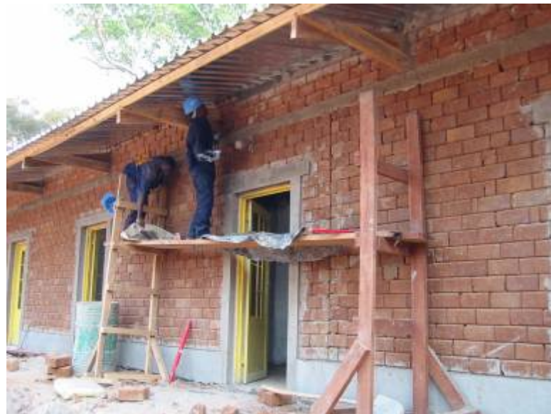
Kinsevere mine contractors' accommodation units under construction. Bricks made on site. (photo Sept 15, 2006)
