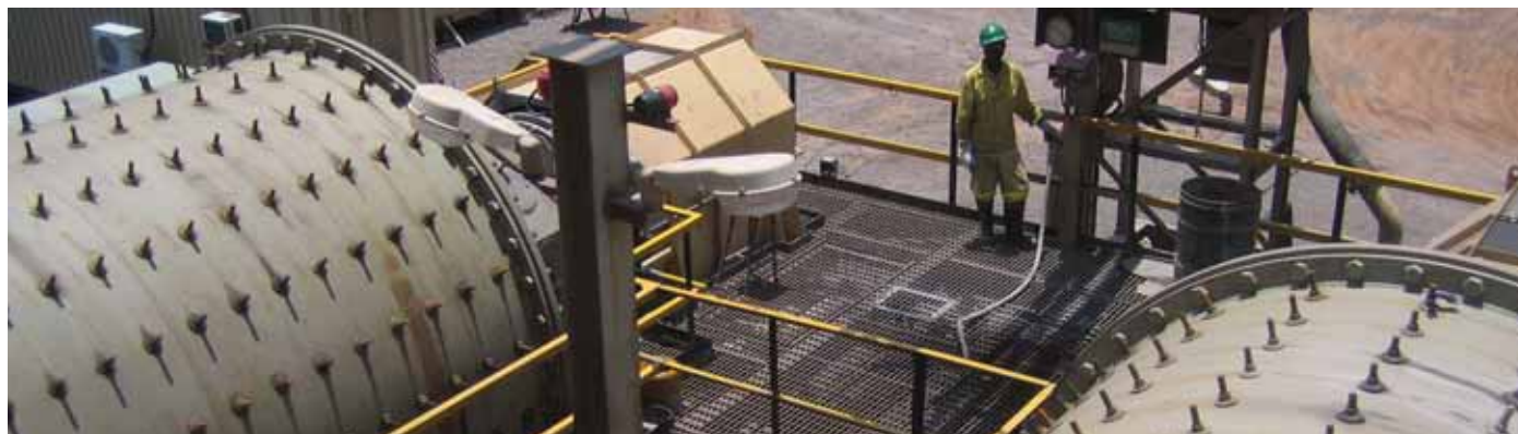
Ball mills at the Dikulushi plant
