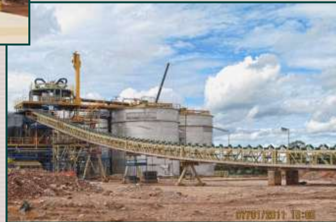
Mill Feed Conveyor Cyclones and Leach tanks
