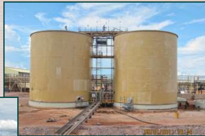
Acid Storage Tanks
