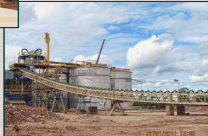
Mill Feed Conveyor Cyclones and Leach tanks
