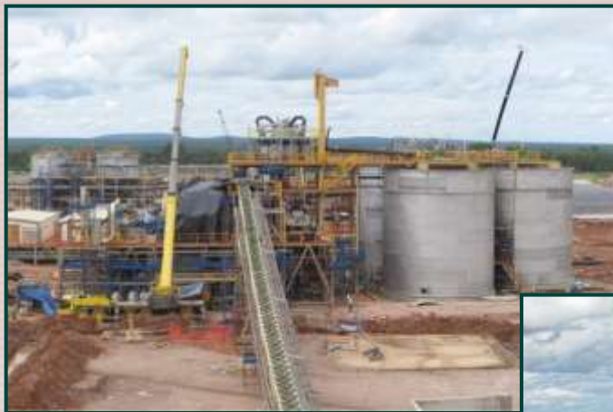
Mill Feed Conveyor Leach Tanks
