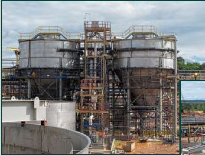
Pin Bed Clarifiers
