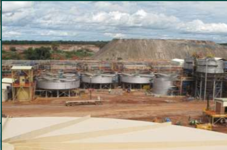
CCD Tanks & Pin Bed Clarifiers (right)
