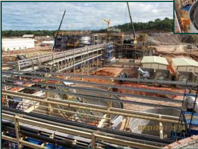
20 Mill, Cyclones & Leach
