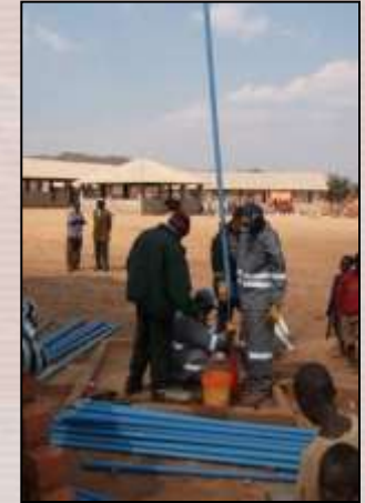
Piping for fresh water well
