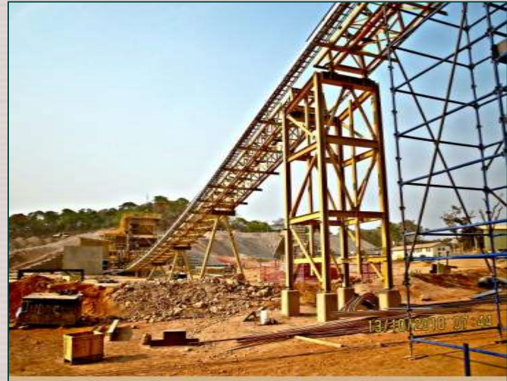
AREA 10 CRUSHER CONVEYOR SYSTEM
